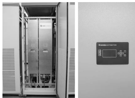
Fig. 9. a,b F3E DA cabinet construction details, F3E DA Control Unit OP
